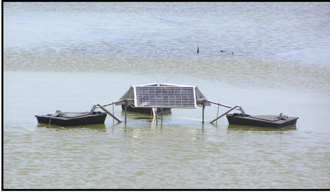
Figure 3-3: Installed Solar Circulator
