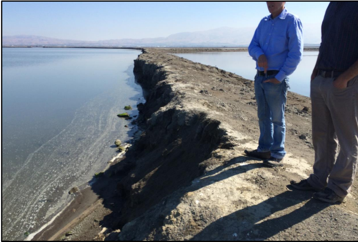
Existing Unengineered Pond Dikes
